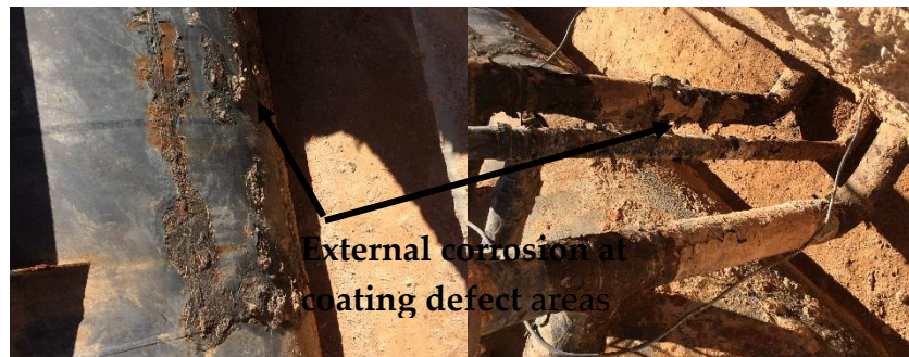
Figure 2: Underground tank and connected pipelines external corrosion
