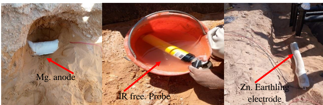
Figure 5: CP system equipment Mg. Anode, Permanent RE and Zn Earthling electrode installation steps
