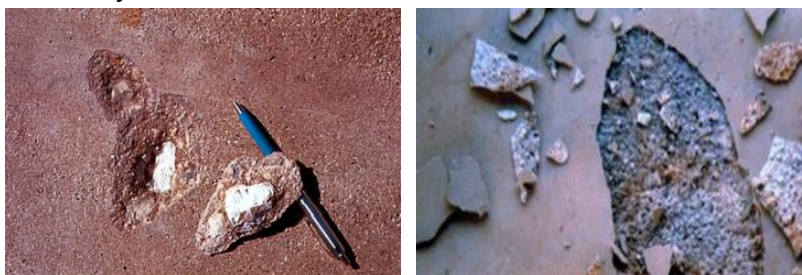
Figure 1: Popout on the slab's surface (left); slab delamination (right) [3].
