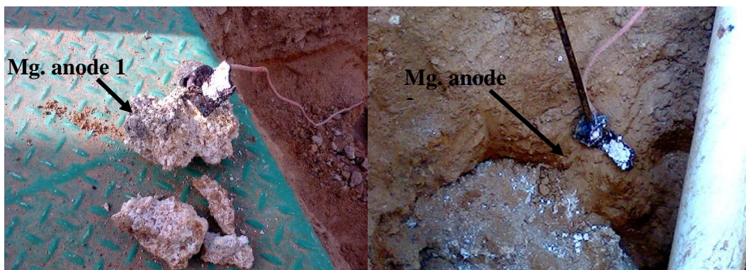
Figure1: Compactly depleted sacrificial anode deleted magnesium
